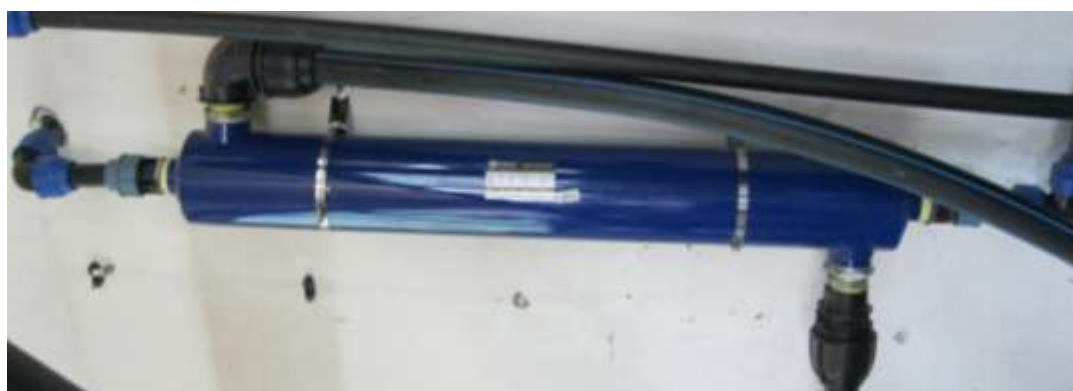
Fig. 4. Water-water heat exchanger for discharging excess heat from the cooling circuit of the generator gas.
