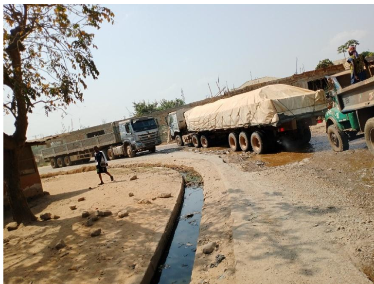
Plate 1: Failed portion of Itori – Ibese Concrete Pavement, commissioned in 2016 (6.936387,3.222095)
