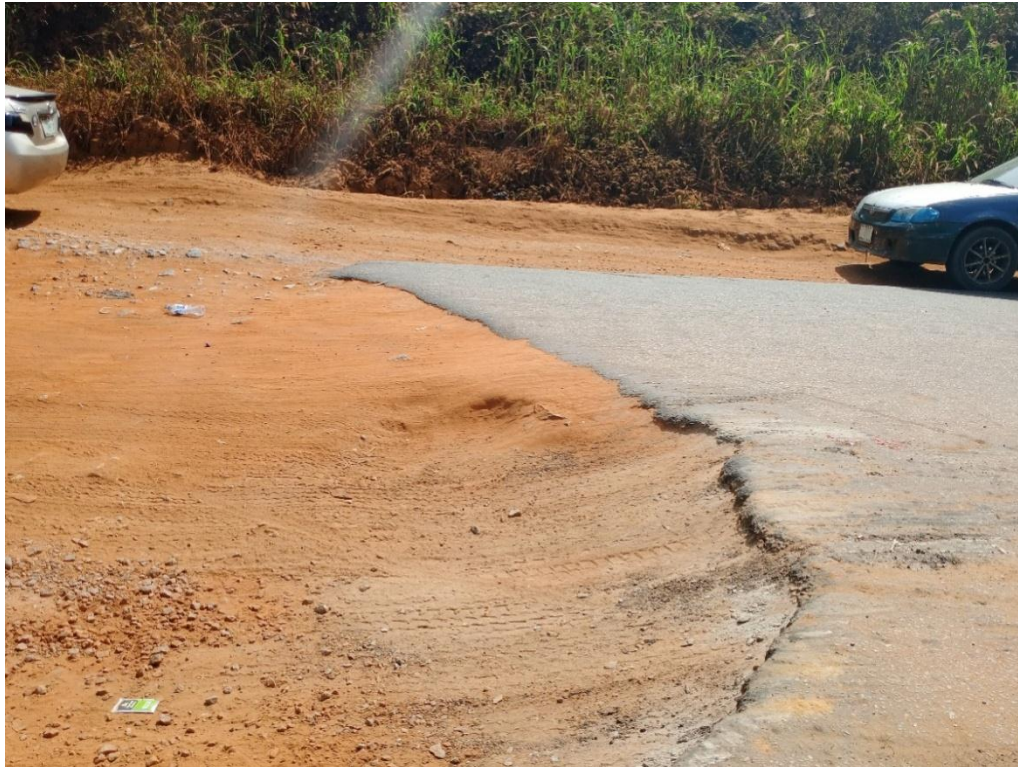
Plate 2: Failed Portion of Ota Abeokuta Asphalt pavement (GPS coordinates: 6.976380, 3.221807)
