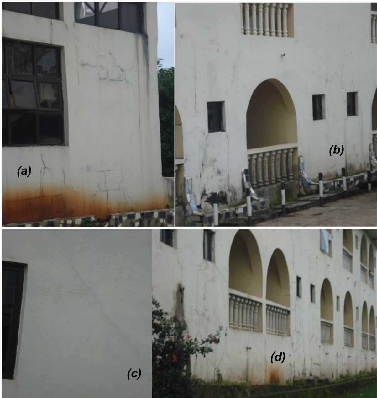
Figure 2: Various parts of the building under study showing some of the cracks observed on it (a) Right, (b) Front, (c) Left and (d) Back
